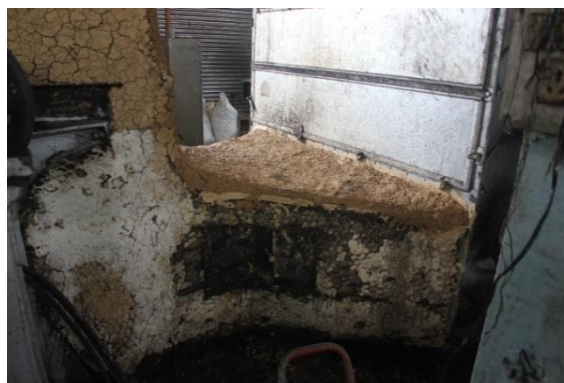
(b) Flue gas passage to heat exchanger
