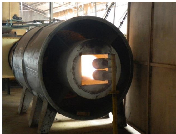
(b) Rear view of a burner
