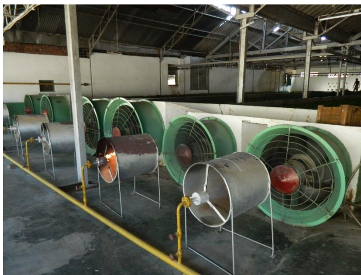
Fig. 5 Gas burner in withering section used at Rupai Tea Factory
