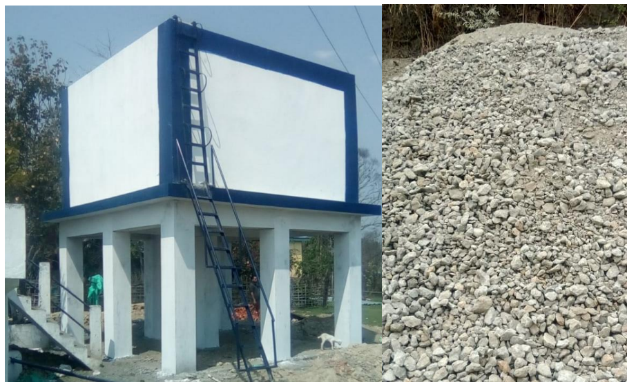
Fig. 2.v.a. Two such Fluoride Nilogon reactors (left) being installed at two 40000 L capacity pipes water supply schemes at Ronkanthir and Kheroni in Karbi Anglong district by PHED Assam. Limestone being collected for the reactors (right)
